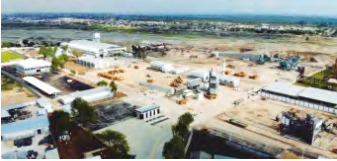
HOT MIXED ASPHALT PLANT, TASHKENT-UZBEKISTAN
