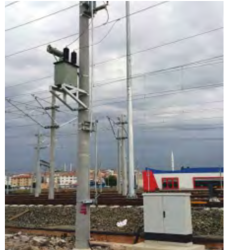
ANKARA HIGH SPEED LINE STATION POINT HEATING SYSEM ANKARA-TÜRKİYE
