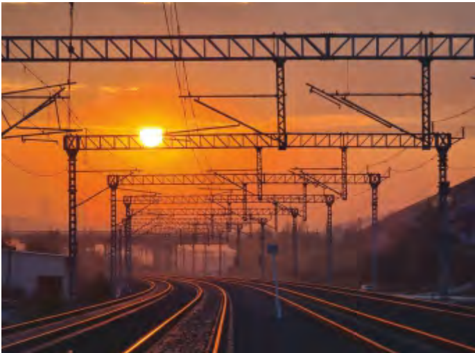
KAYAŞ-YERKÖY HIGH SPEED TRAIN LINE, CATENARY SYSTEM, ANKARA-YERKÖY-TÜRKİYE
