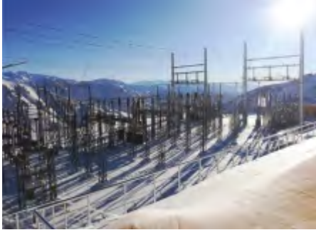
SALANG TUNNEL SUBSTATION (220 KV) AND NETWORK (20 KV)-AFGHANISTAN
