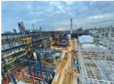
MOSCOW REFINERY-SULPHUR RECOVERY UNIT (SRU) THE RUSSIAN FEDERATION
