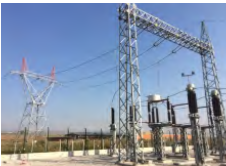
BANDIRMA-MENEMEN RAILWAY ELECTRIFICATION SUBSTATIONS (154 KV), BALIKESİR-TÜRKİYE
