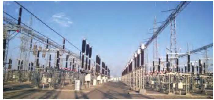
AHAL-2 SIMPLE CYCLE GAS TURBINE POWER PLANT (252,2 MW, 220 KV/110 KV SWITCHYARD) TURKMENISTAN
