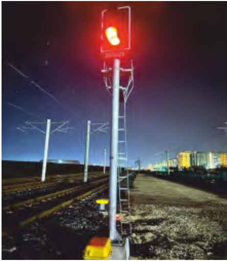
GAZİRAY HIGH SPEED TRAIN AND COMMUTER LINE, SIGNALING AND TELECOMMUNICATION SYSTEMS, GAZİANTEP-TÜRKİYE
