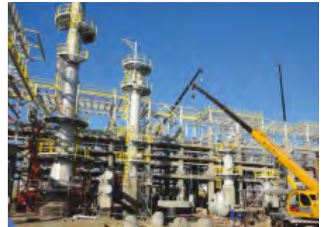
AZERIKIMYA EP300 ETHYLENE PLANT SUMQAYIT-AZERBAIJAN
