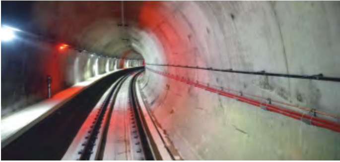
SABİHA GÖKÇEN AIRPORT METRO LINE ELECTRICAL WORKS, İSTANBUL-TÜRKİYE
