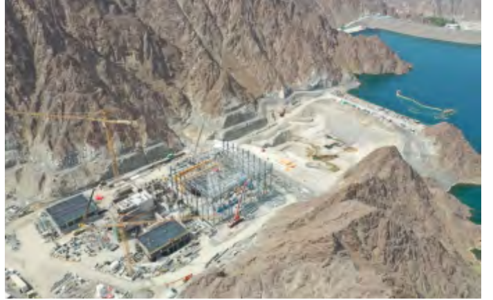
HATTA PUMPED STORAGE HYDRO POWER PLANT, DUBAI-UAE
