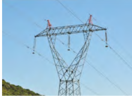
KIŞLADAĞ GOLD MINE SUBSTATION (154 KV), UŞAK OSB SUBSTATION ENERGY TRANSMISSION LINE (28 KM)-TÜRKİYE
