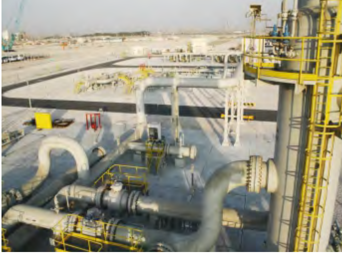
MESSAID CONSUMERS GAS SUPPLY PLANT-QATAR
