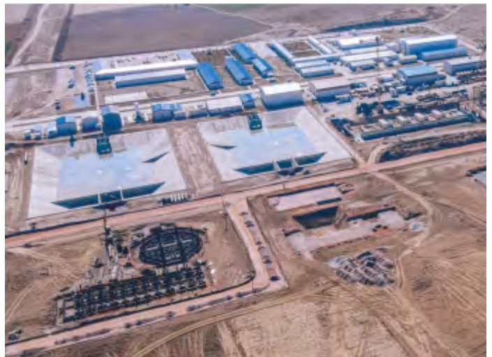
TUZ GÖLÜ UNDERGROUND NATURAL GAS STORAGE PLANT, AKSARAY-TÜRKİYE
