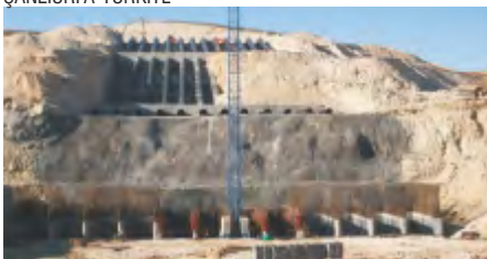
SURUÇ PLAIN IRRIGATION PUMP STATION AND TRANSMISSION FACILITIES, ŞANLIURFA-TÜRKİYE
