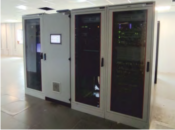
MARMARAY CR3 TELECOMMUNICATION SYSTEMS AND MAINTENANCE, İSTANBUL-TÜRKİYE
