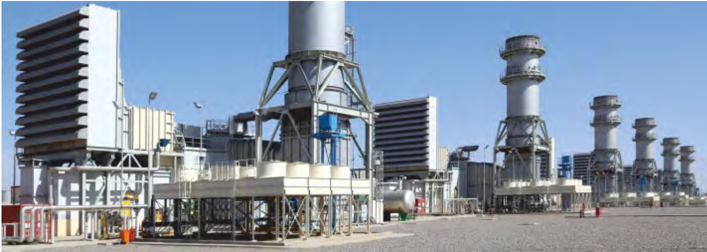
NAINAWA SIMPLE CYCLE POWER PLANT-IRAQ
