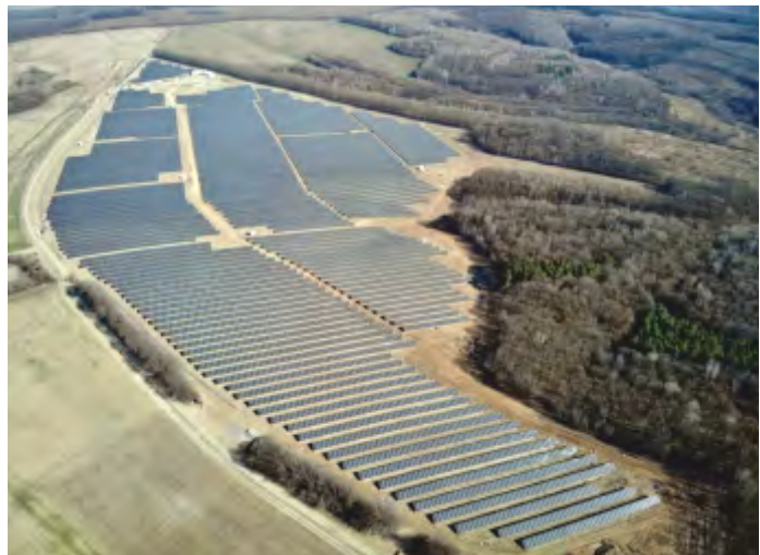
HATNA SOLAR POWER PLANT (24 MW), KHMELNYTSKYI-UKRAYNA
