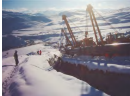
BAKU-TBİLİSİ-CEYHAN (BTC) CRUDE OIL PIPELINE LOT-8 PORTION-TÜRKİYE
