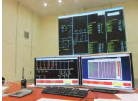
NATIONAL LOAD CONTROL CENTER (NLCC) KABUL-AFGHANISTAN
