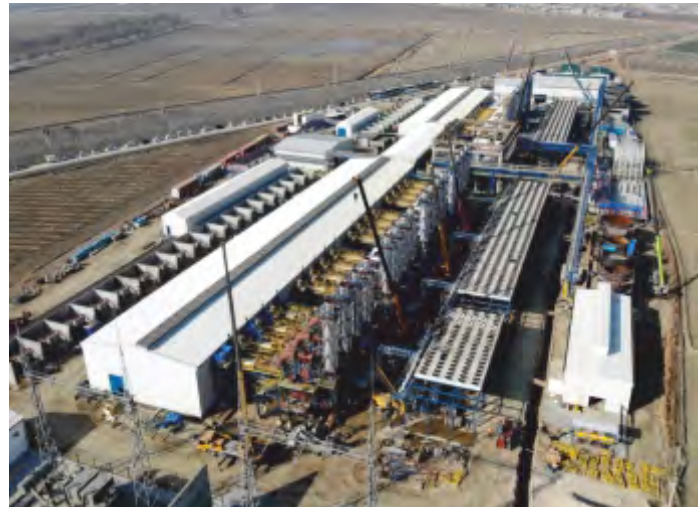
NATURAL GAS CONVERSION PLANT, BUHARA-UZBEKISTAN
