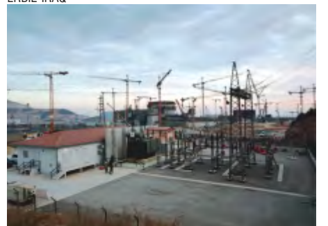
AKKUYU NUCLEAR POWER PLANT TEMPORARY SUBSTATION (154 KV), MERSİN-TÜRKİYE
