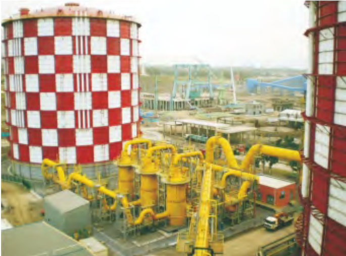
İSDEMİR BLAST FURNACE AND CONVERTER GASES STORAGE PLANT, İSKENDERUN-TÜRKİYE
