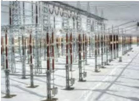
VAN SUBSTATION (380 KV)-TÜRKİYE
