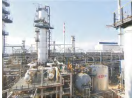
DIESEL KEROSENE HYDR PROCESS AND CCR REFORMER IZMIT, KOCAELİ-TÜRKİYE
