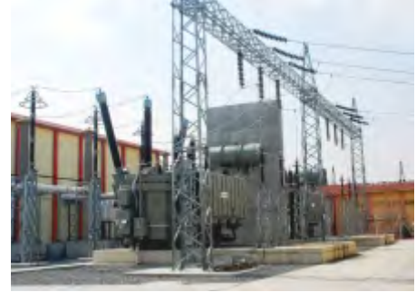
YENİBOSNA GIS SUBSTATION (420 KV), İSTANBUL-TÜRKİYE
