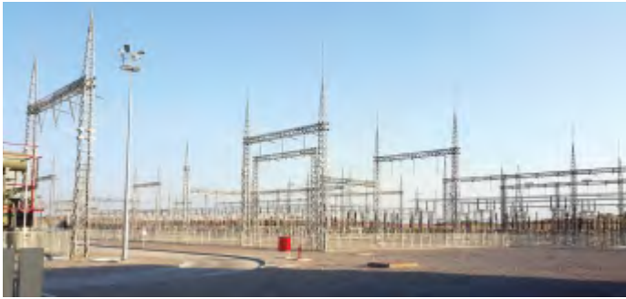
DERWEZE SIMPLE CYCLE GAS TURBINE POWER PLANT (504,4 MW, 220 KV/110 KV SWITCHYARD) TURKMENISTAN
