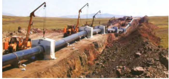
SAMSUN-ANKARA NATURAL GAS PIPELINE-TÜRKİYE
