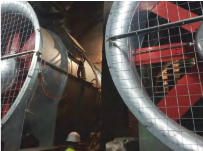
TBILISI METRO VENTILATION SYSTEM, TBILISI-GEORGIA
