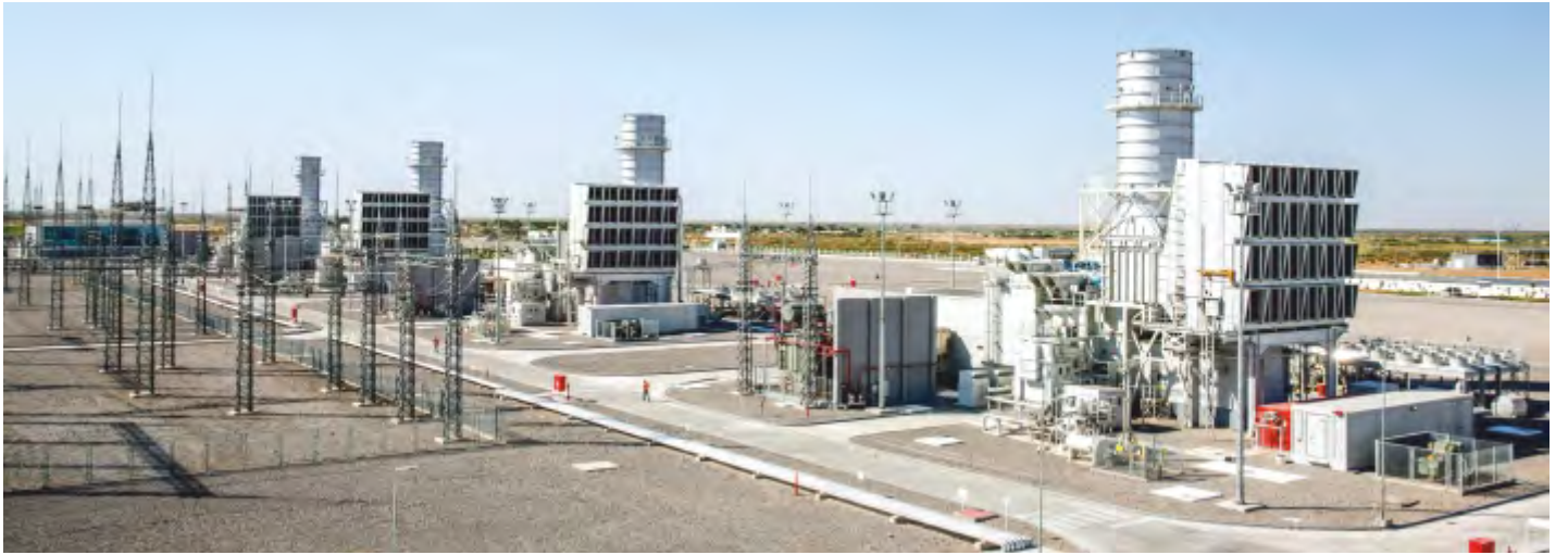
DERWEZE SIMPLE CYCLE POWER PLANT-TURKMENISTAN
