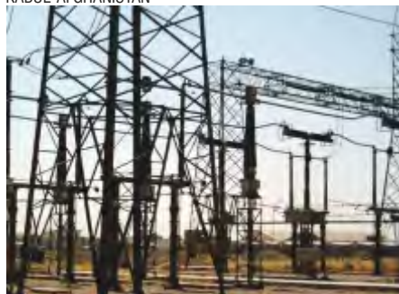
BAIJI GAS POWER PLANT UPGRADE PROJECT SWITCHYARD (400 KV)-IRAQ
