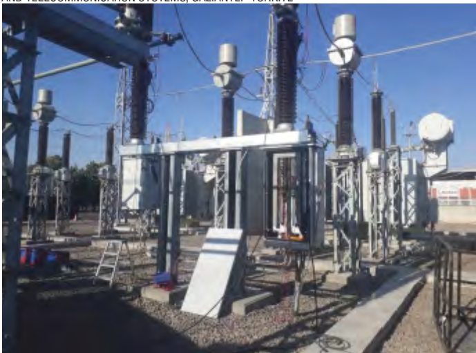
GAZİRAY TRANSFORMER STATION, GAZİANTEP-TÜRKİYE
