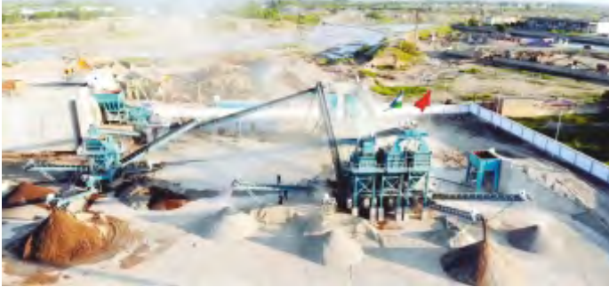
AGGREGATE CRUSHING AND SCREENING PLANT, TASHKENT-UZBEKISTAN
