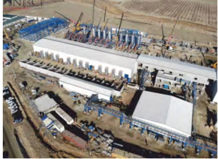
NATURAL GAS CONVERSION PLANT, BUHARA-UZBEKISTAN
