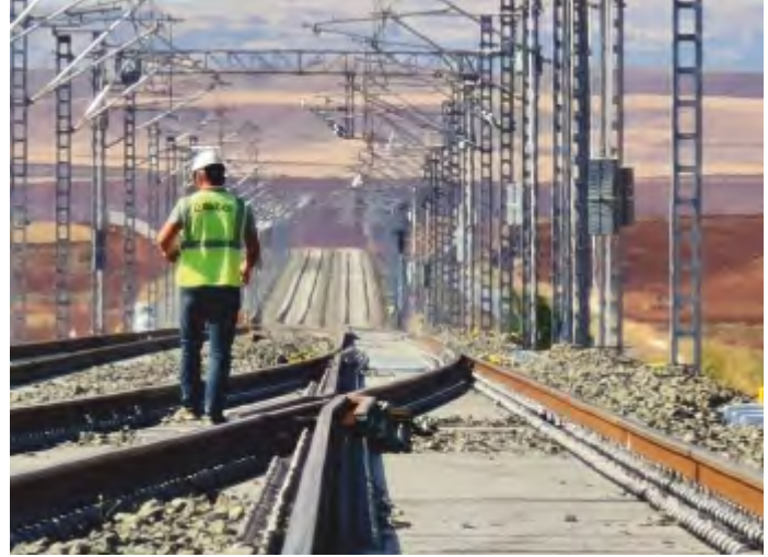
KAYAŞ-YERKÖY HIGH SPEED TRAIN LINE, SIGNALING AND TELECOMMUNICATION SYSTEMS ANKARA-YERKÖY-TÜRKİYE
