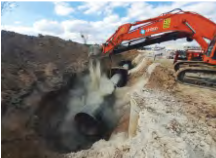
ASKI WATER SUPPLY PIPELINE (İVEDİK-TEMELLİ-POLATLI) RESERVOIRS, PUMP STATIONS FACILITIES, ANKARA-TÜRKİYE
