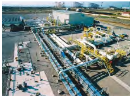
GARADAG GAS COMPRESSOR STATION-AZERBAIJAN
